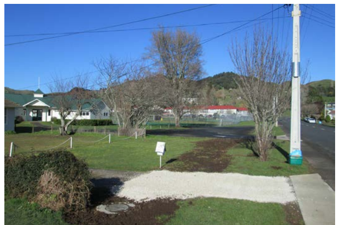
A section of new 500mm concrete pipe was installed to replace the old 200mm pipe. Better storm water drainage is provided with new manholes.
